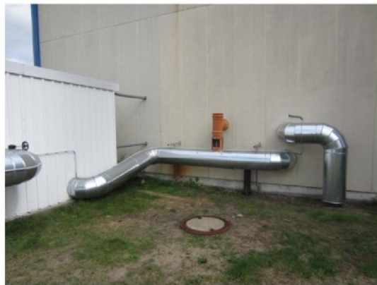
C) Dosing point at the thermal water cycle
